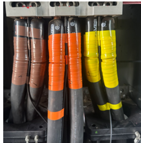
Figure 11 - Sensors attached directly to insulated cables
